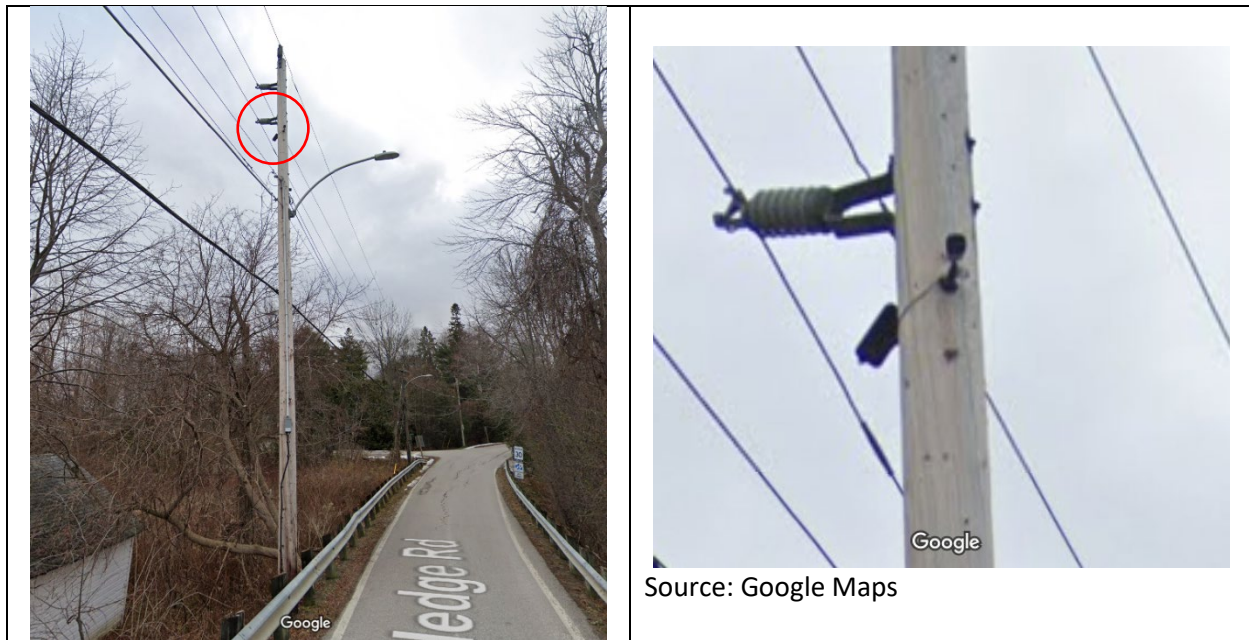
Figure 6: Mounted Camera for Mossington Bridge Surveillance
