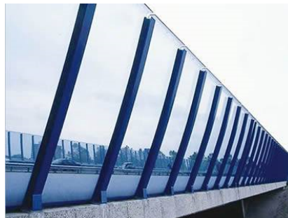
Figure 1 – Acrylic barrier on the parapet of a bridge.
