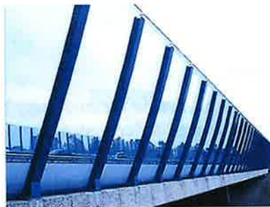
Figure 1 – Acrylic barrier on the parapet of a bridge.
