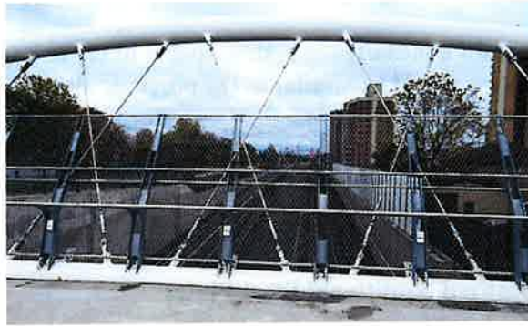
Figure 2 – Localized fencing around structural members
